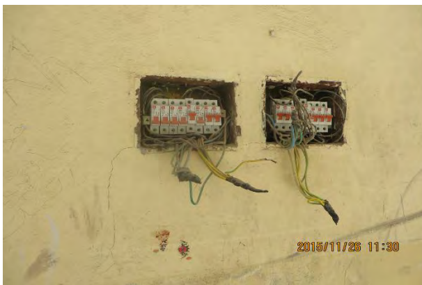
Photo 7 – Exposed Circuit Breakers at Educational Facility S145A
