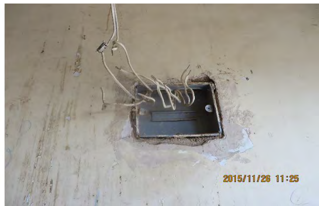
Photo 8 – Exposed Wiring in an Electrical Box at Educational Facility S145A
