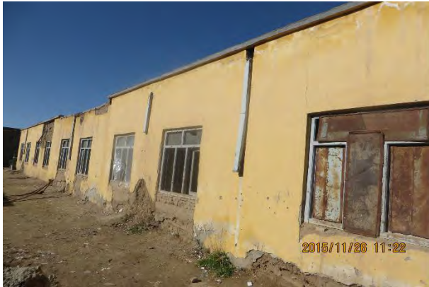
Photo 5 – Missing Downspouts at Educational Facility S145A
