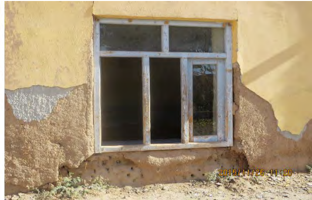
Photo 6 – Plaster Failure at Educational Facility S145A
