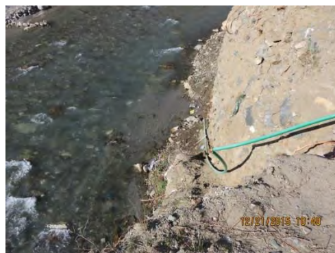
Photo 2 - Water Hose Delivering Untreated River Water to the Hospital
