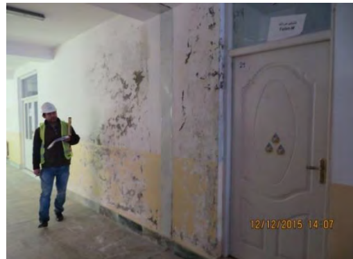
Photo 3 - Mold on the First-Floor Corridor Wall
