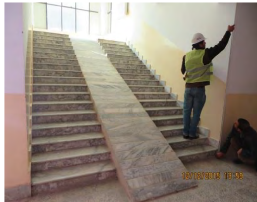
Photo 4 - The Stairway Lacks Handrails, and the Wheelchair Ramp's Slope Remains Excessive
