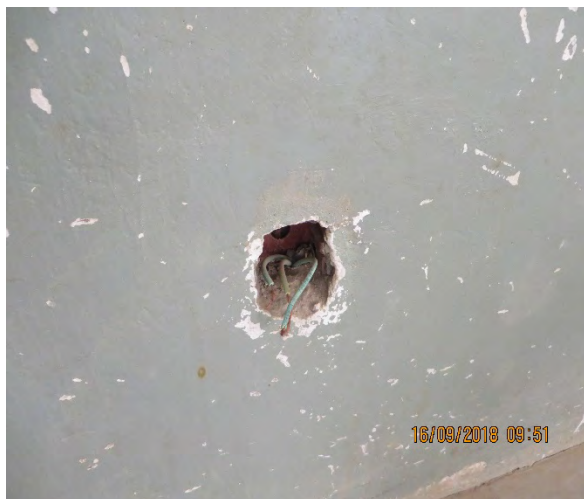
Photo 5 - Exposed Wires at School S046B
