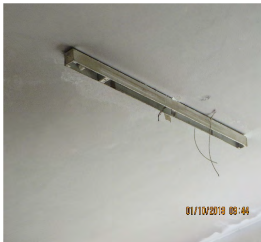
Photo 6 - Broken Lights at School S053A
