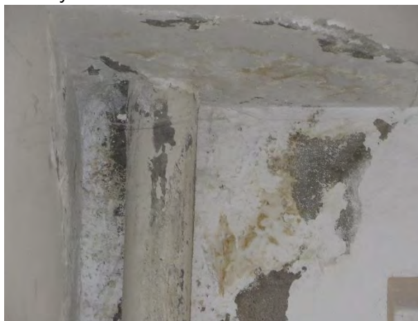
Photo 2 - Evidence of leaking roof at Facility 751
