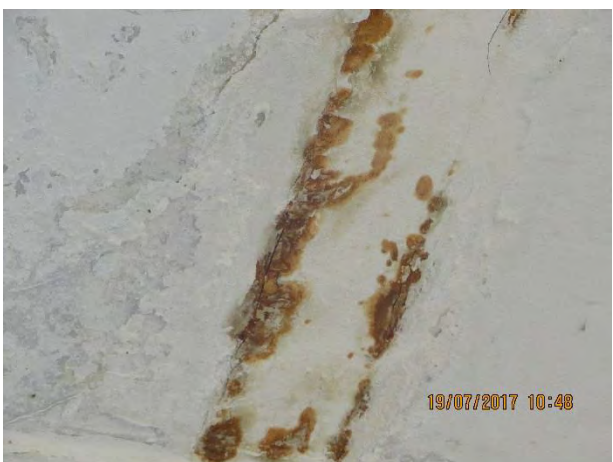
Photo 3 - Mold and leakage at Facility 2963
