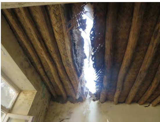
Photo 6 - Ceiling and Structural Damage at School SR02
