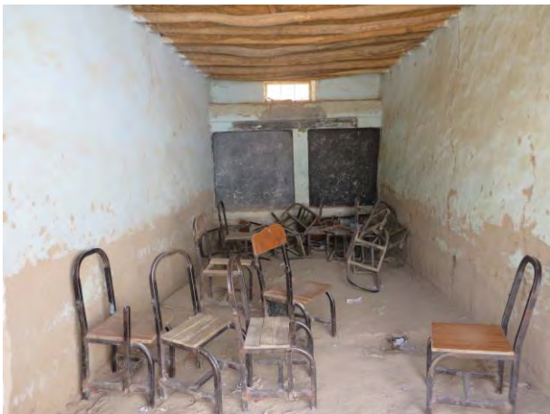
Photo 10 - Broken furniture pile at School SR03
