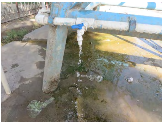
Photo 4 – Water tank at School S228A in Kunduz City
