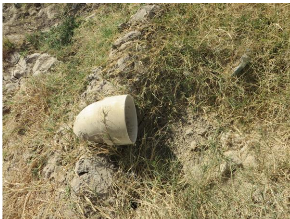
Photo 4 – Incomplete Water Pipe Protruding from Unlevelled Football Field
