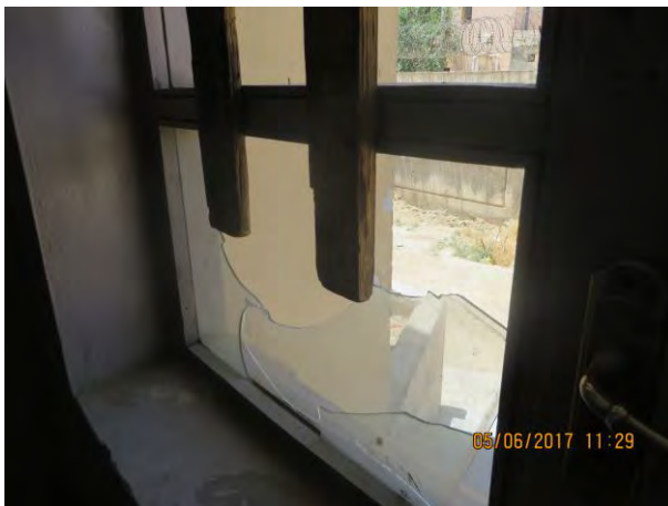
Photo 7 - Broken windows at School S173A
