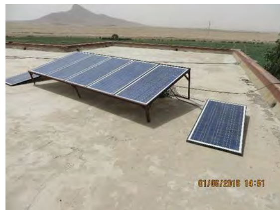
Photo 12 - Solar Panels at Facility 735
