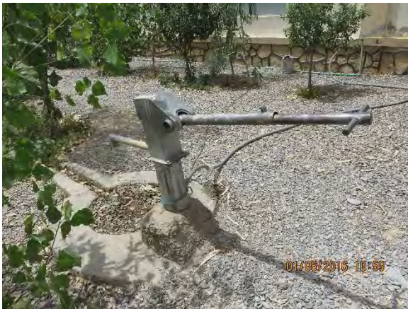
Photo 9 – Water Well at Facility 735
