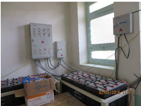
Photo 7 - Facility 747's Electrical Equipment
