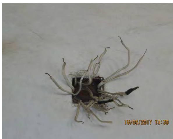
Photo 3 - Exposed Wires at School S076A in Maymana
