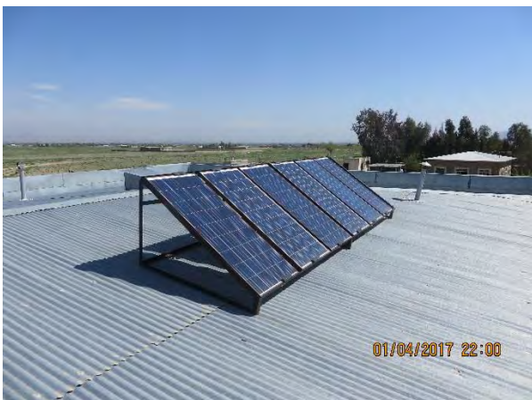
Photo 1 - Solar Panels at Facility 866
