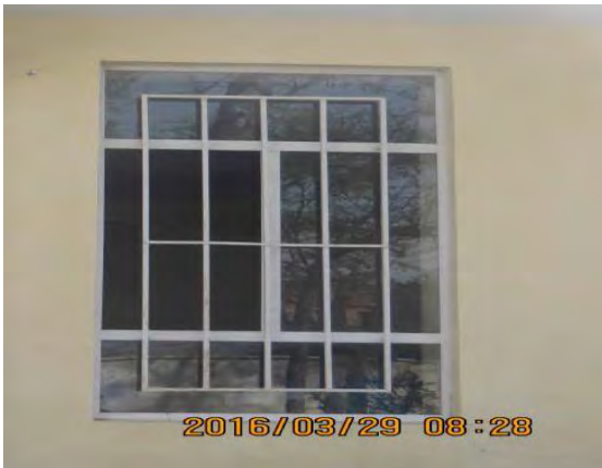
Photo 7 – Missing Windows at SKP-3 in Hisa e Awal Kohistan
