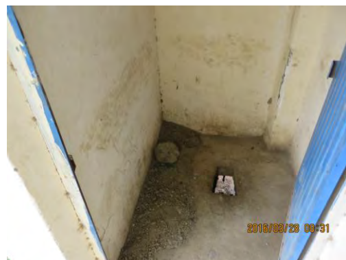
Photo 6 - Uninsulated Toilet Pit in SKP-1 at Hisa e Awal Kohistan
