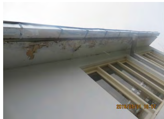
Photo 9 – Water Damage to Underside of Roof at SKP-6 in Nejrab
