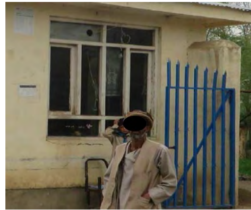
Photo 8 – Broken Windows at SKP-1 in Hisa e Awal Kohistan
