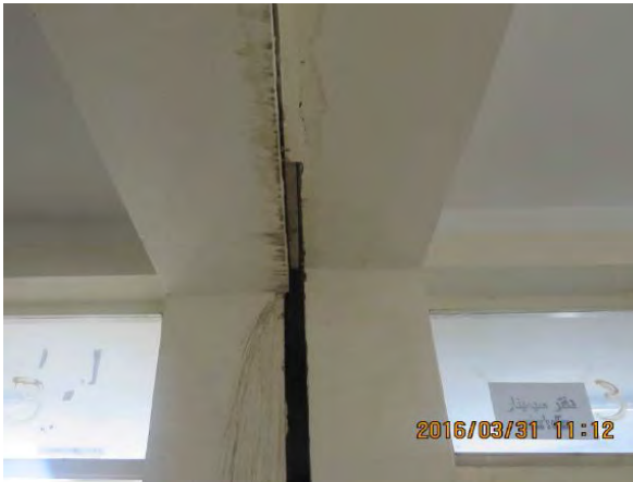
Photo 10 – Mold on Hallway Ceiling at SKP-5 in Nejrab
