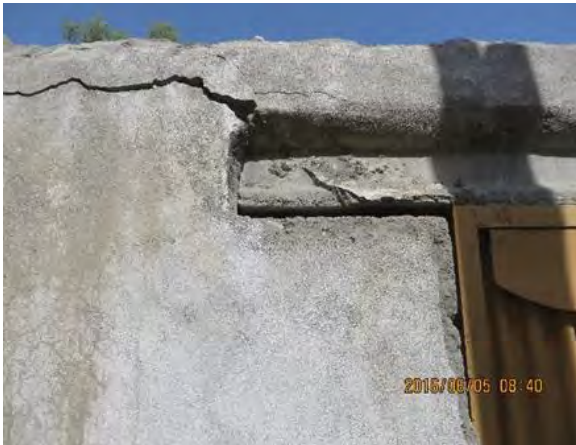
Photo 13 - External Crack at Health Facility 307
