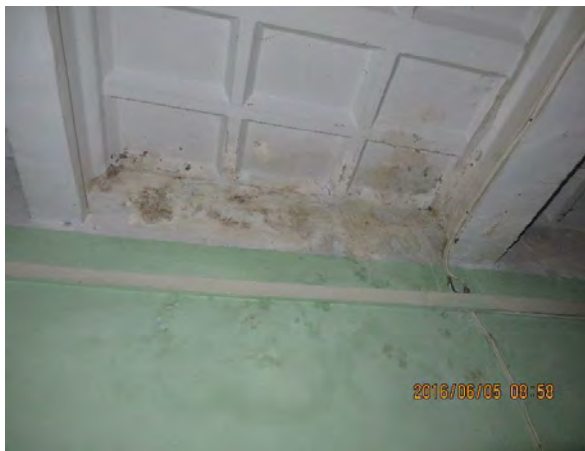
Photo 15 - Possible leak or mold at Health Facility 307
