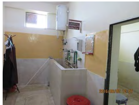
Photo 10 - Hand Washing Station at Health Facility 2676
