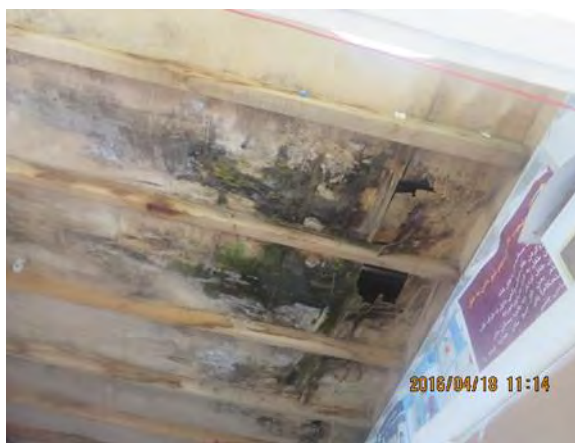
Photo 4 - Damage at Facility 2386
