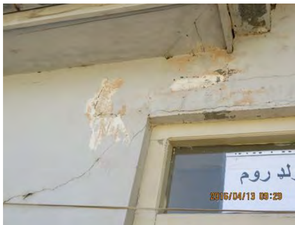
Photo 2 - Cracked Walls at Facility 434
