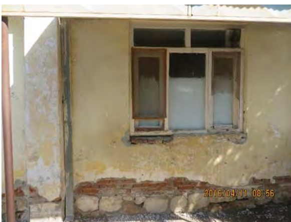
Photo 3 - Damage at Facility 427
