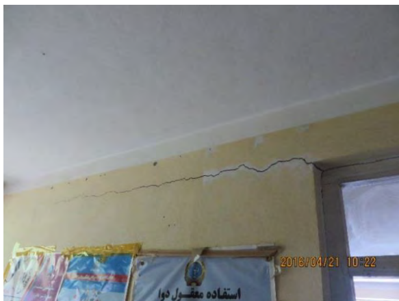
Photo 1 - Cracked Walls at Facility 431
