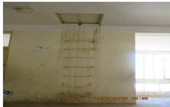
Photo 4 – Apparent Water Damage from Leaks at Azady School
