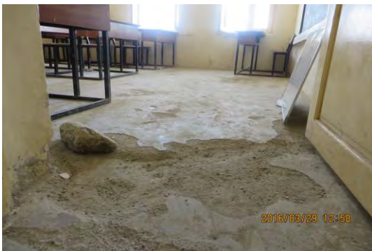
Photo 3 – Damaged Concrete Surface in Classroom at Azady School
