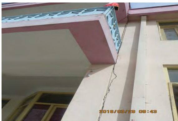
Photo 6 – Crack Running the Vertical Length of Bakhtnoor Bakhtiar School
