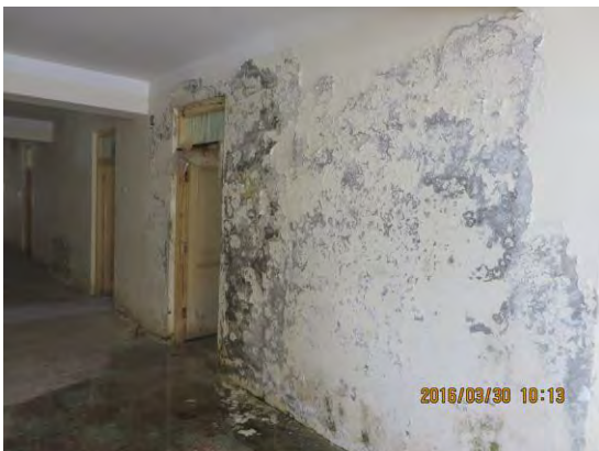
Photo 13 – Damaged Walls and Standing Water Inside the Hostel
