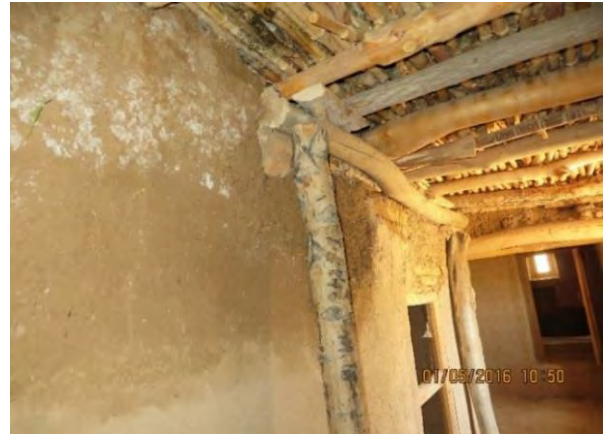
Photo 4 – Leaking Roof and Saturated Walls at Health Facility 2616
