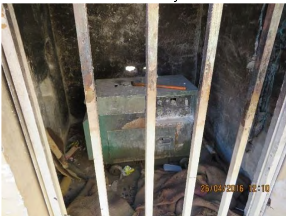
Photo 1 - Damaged and Inoperable Generator at Health Facility 2039
