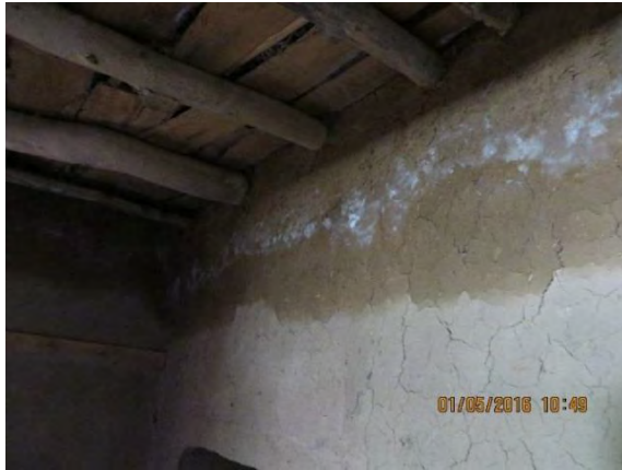
Photo 3 - Leaking Roof and Saturated Walls at Health Facility 2616
