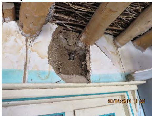
Photo 2 - Structural Damage at Health Facility 2476
