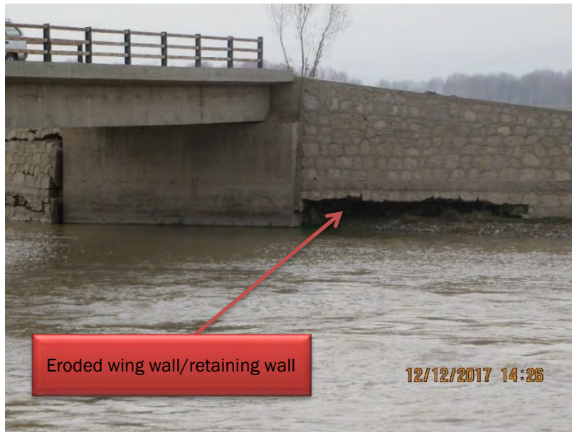
Photo 1: Eroding Bridge Wall
