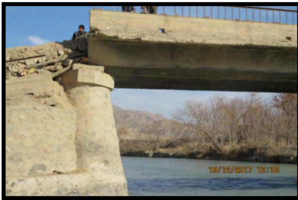
Photo 1: Structural Deterioration of the Bridge Poses Safety Risks
