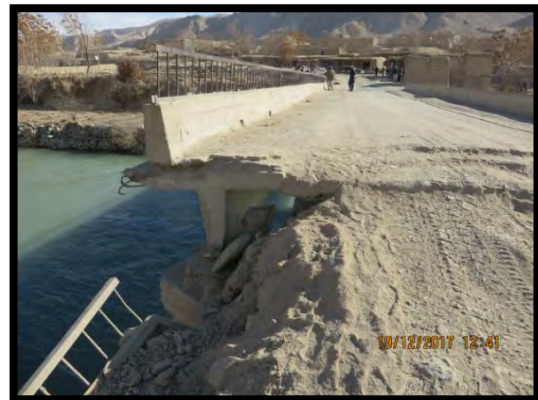
Photo 2: Structural Deterioration of the Bridge Poses Safety Risks
