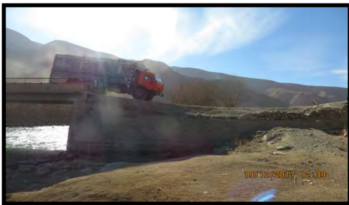
Photo 3: Cracks in Bridge Foundation and Elevation Difference from Bridge to Road
