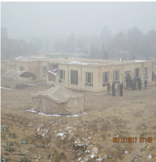
Photo 1: Outside of SR-09 Showing Significant Blast Damage
