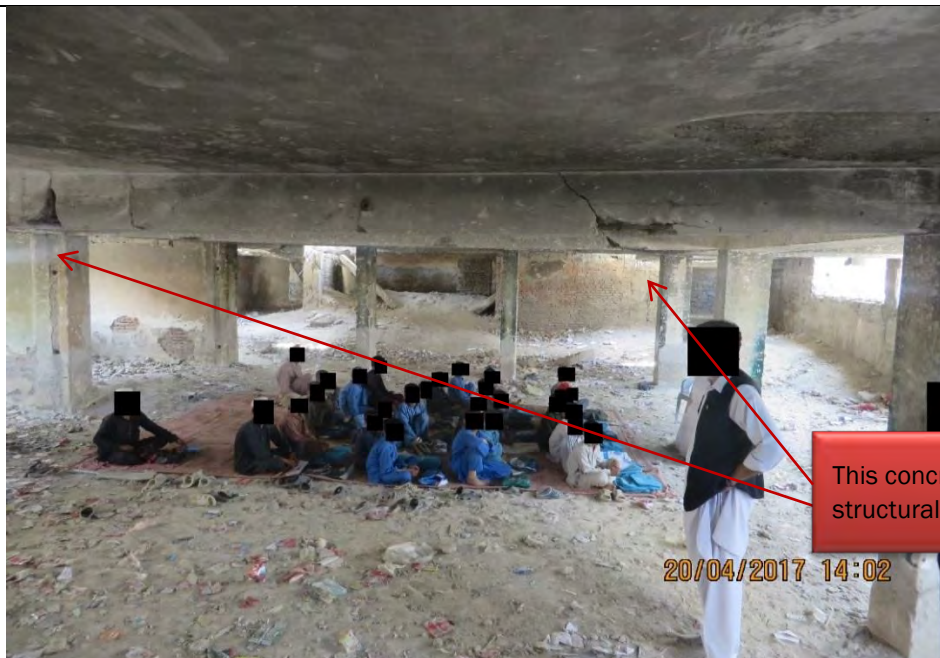
Photo 2: Unrepairable Damage to Building near SR 21 Being Used as a Classroom
