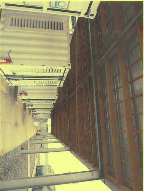
USAID Built Diesel Plant at SPS
