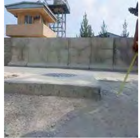
An improperly built manhole which poses a safety hazard to motorists. (SIGAR photo)
