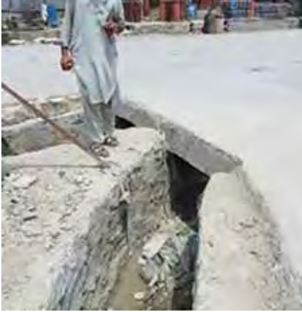
Ghulam Khan road culvert missing required protective walls. (SIGAR photo)
