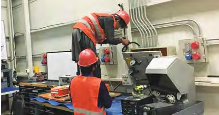
Two Afghan quality-assurance employees inspecting a fuse box at a USACE construction project. (SIGAR photo)
