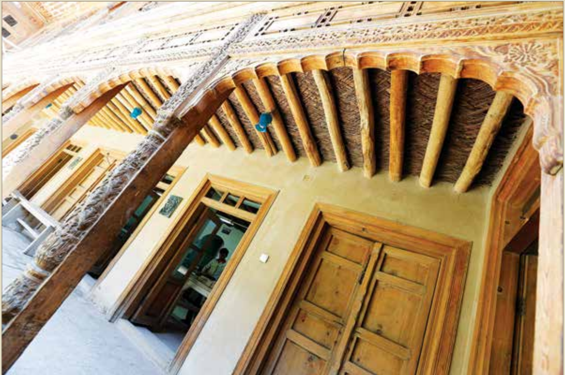
Despite the war, these buildings in the Murad Khani district of Kabul are being restored to their 18th-century character and intricate wood work. (UNAMA photo by Fardin Waezi)
