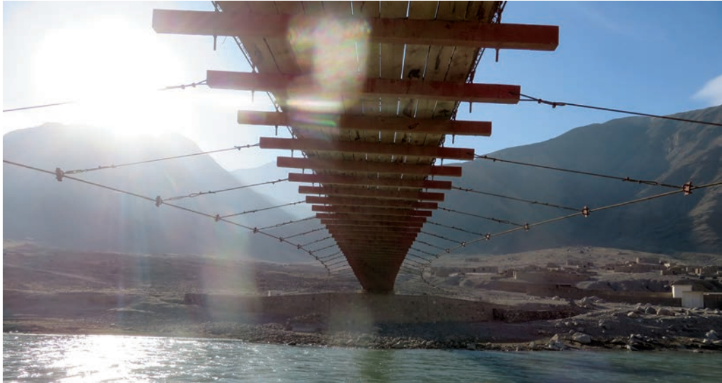
A DOD-funded pedestrian bridge crosses a river in Baghlan Province. (SIGAR photo)
