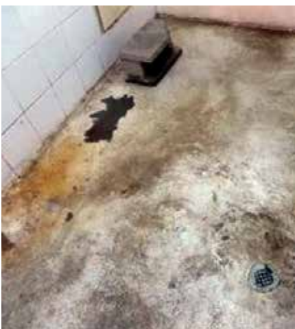
Improperly sloped shower floor with mold in one officers' barracks. (SIGAR photo)
