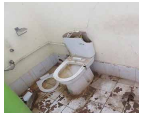
Broken toilet in the guard quarters building of Wardak Prison. (SIGAR photo)
