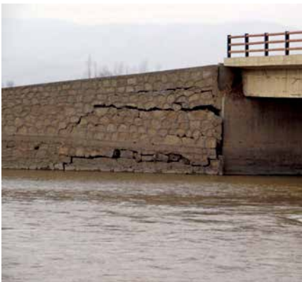
Severe cracks in a Baghlan Bridge retaining wall. (SIGAR photo)
