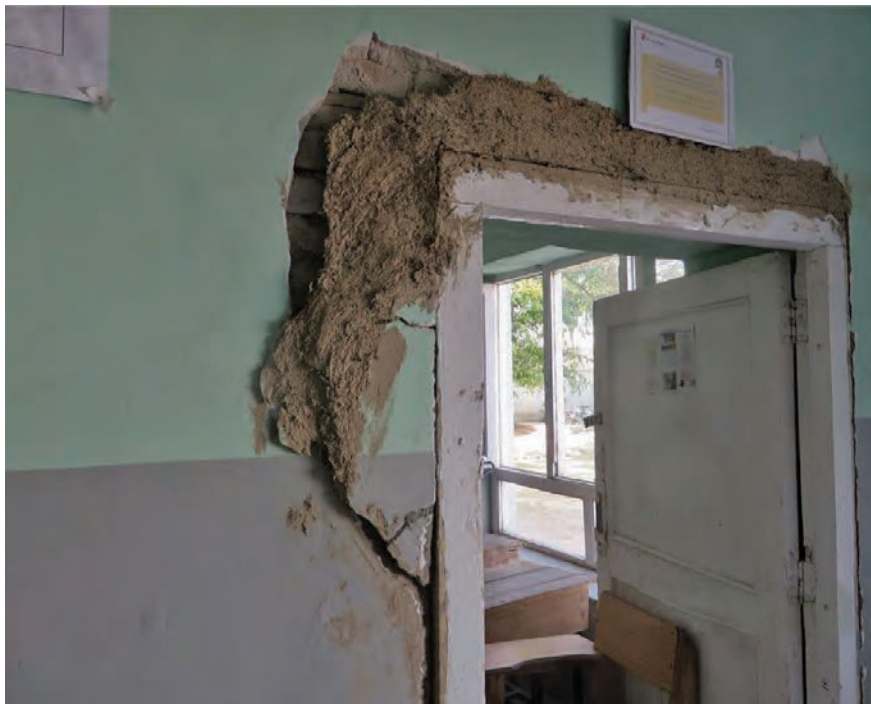
Structural damage at a school in Faryab Province. (SIGAR photo)
