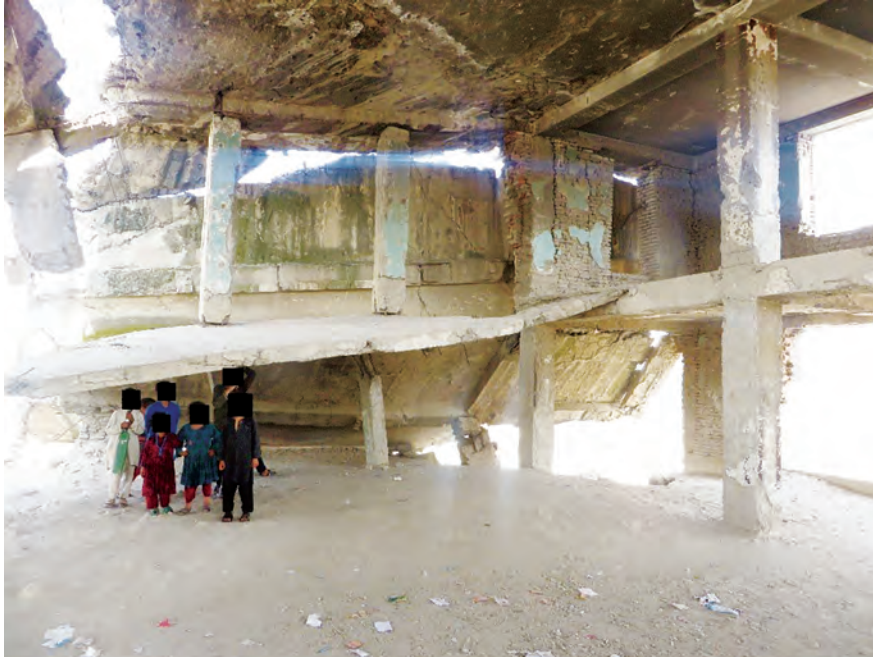
Irreparable damage to building used as a classroom in Khowst Province. (SIGAR photo)
