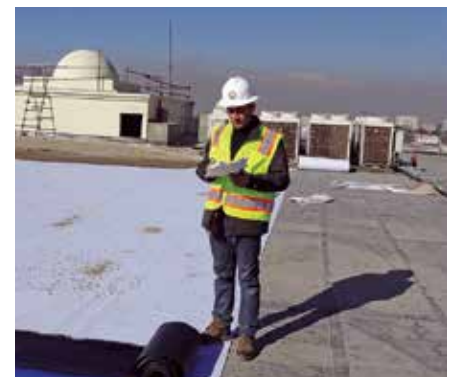
A SIGAR inspector checks work at the new Afghan Ministry of Defense headquarters. (SIGAR photo)
