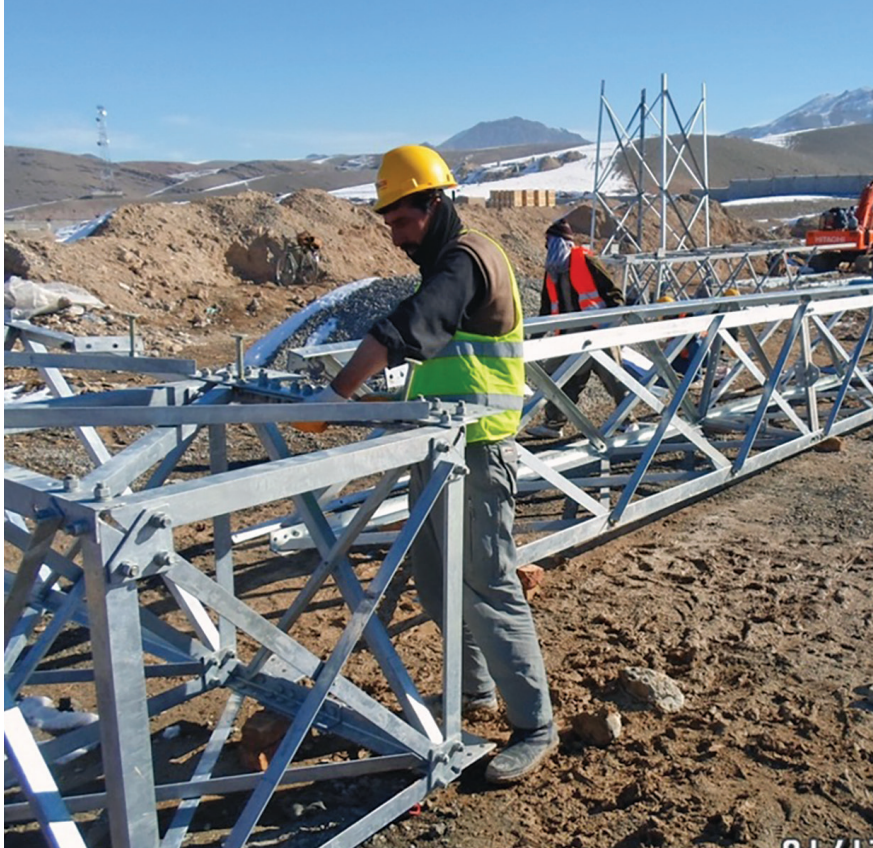
Workers assemble a tower for an electrical project to connect regional transmission systems. (USAID photo)
