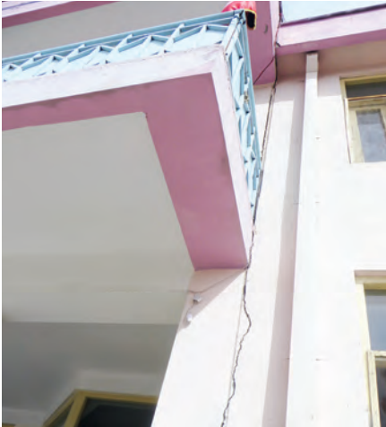
Vertical crack in the facade of Bakhtnoor Bakhtiar School, Khowst Province. (SIGAR photo)
