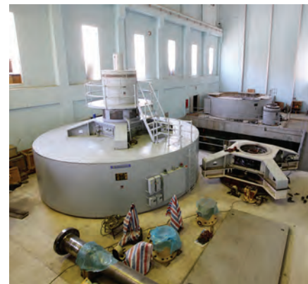
The turbine hall at Kajaki Dam. (UK Ministry of Defence photo by SGT Anthony Boocock)
