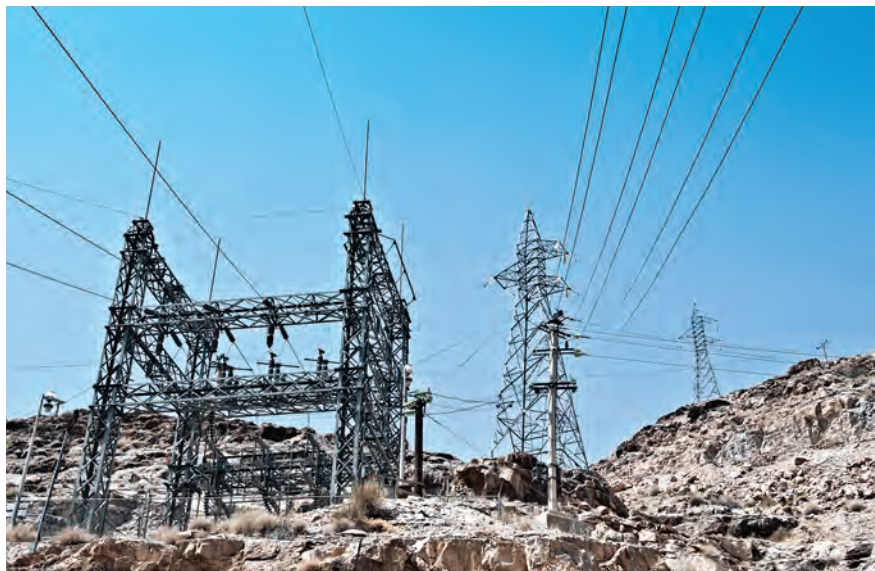
A substation and power lines on rugged hills by the Kajaki Dam are part of the infrastructure needed to expand electric service in Afghanistan. (U.S. Navy photo by Specialist 2nd Class Jonathan David)
