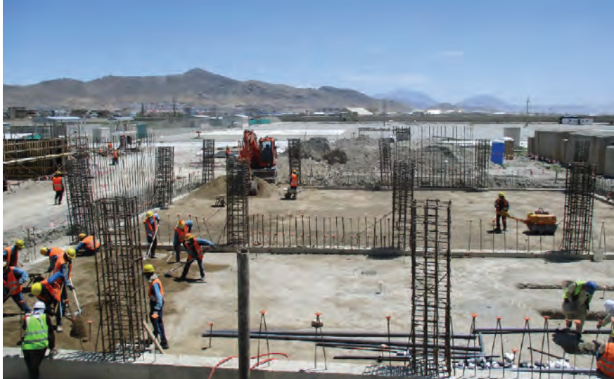
MOI Headquarters, Women's Compound Fitness Facility, in Kabul Province (CSTC-A CJ-Eng photo)
