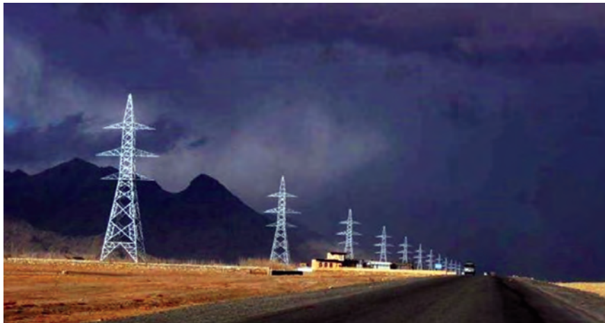
Transmission towers along the Arghandi-Ghazni line, part of more than 500 km of USAID-supported construction to connect power systems from Kabul to Kandahar and Helmand. (USAID photo)
