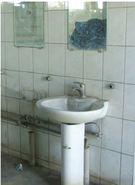
Poorly maintained facilities in bathroom at Afghan Air Force University, March 2015. (SIGAR photo by Aziz Zaki)
