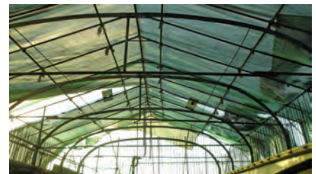
Interior view of a magazine under construction in Kabul Province. (USACE-TAA photo)
