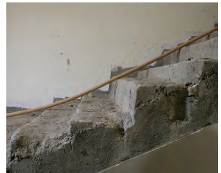
Crumbling stairs of varying heights at Garm Ser ANP District Headquarters, June 27, 2010. (SIGAR photo)
