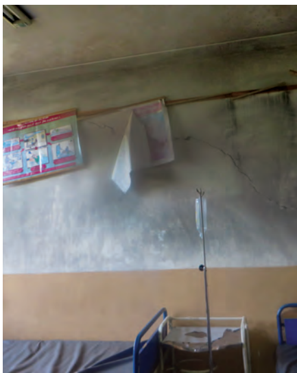
SIGAR's site inspections of health facilities in Kabul revealed basic structural concerns at most facilities, such as cracked walls. (SIGAR photo)
