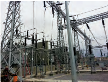
IRD provided quality-assurance services for this new power substation in Kandahar. IRD's contract with USAID was the subject of a SIGAR financial audit this quarter. (USAID photo)
