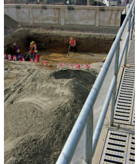
Over-excavation of sewage filter beds. (SIGAR photo)
