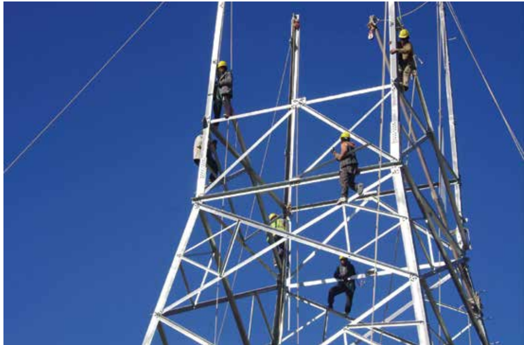
Workers assemble a transmission line tower. The Engineering Support Program provided construction management services and quality assurance for many of USAID's power-infrastructure projects. (USAID photo)
