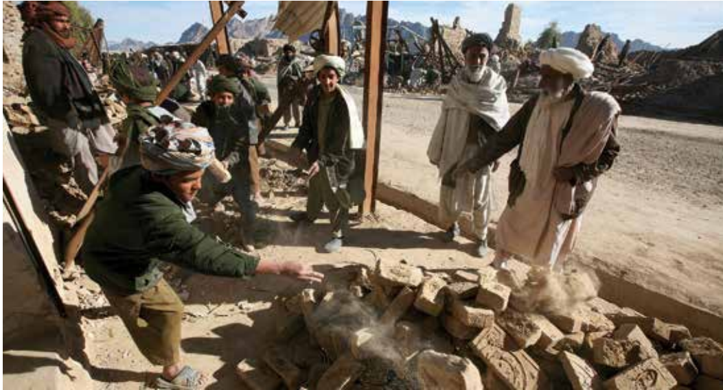
Using CERP funding, Afghan men work on rebuilding market spaces in Helmand Province in late 2009. (U.S. Marine Corps photo)
