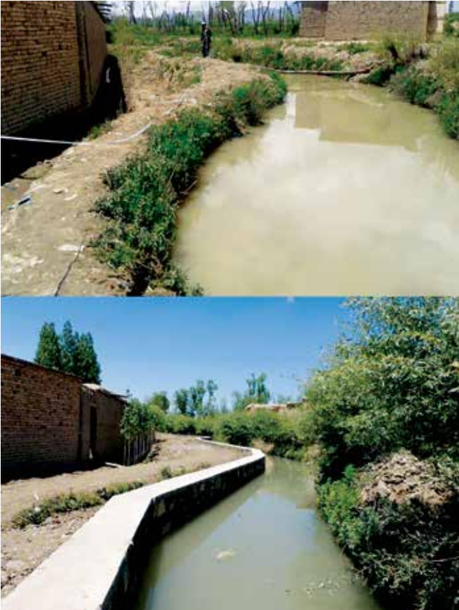
Before and after photographs of a flood protection wall built by USAID in Ahmadabad District, Paktiya Province. (USAID photo)
