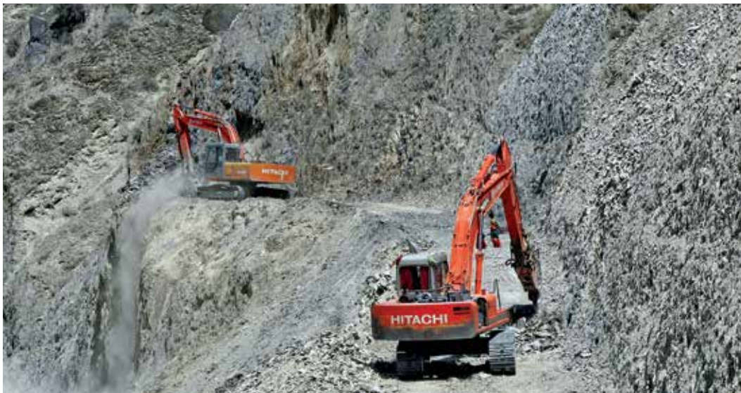
USAID road construction efforts along the Khost-Gardez road in March 2010. (USAID photo)
