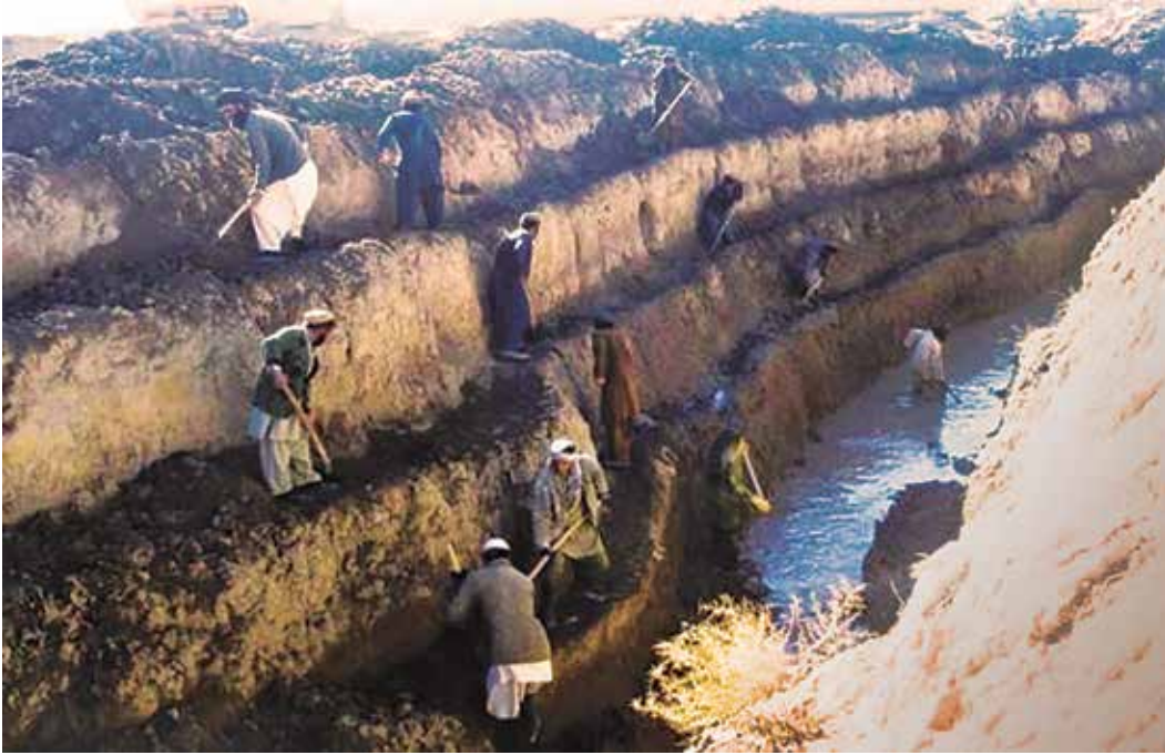
The Abbas Qala Community Development Council used a USAID grant to clear a deep karez (irrigation canal) in Baraki Barak District, Logar Province. Members of three local communities served by the karez terraced one wall and then formed a shovel brigade to move debris from the bottom to the top in November 2013. (Photo by Ahmad Salarzai)
