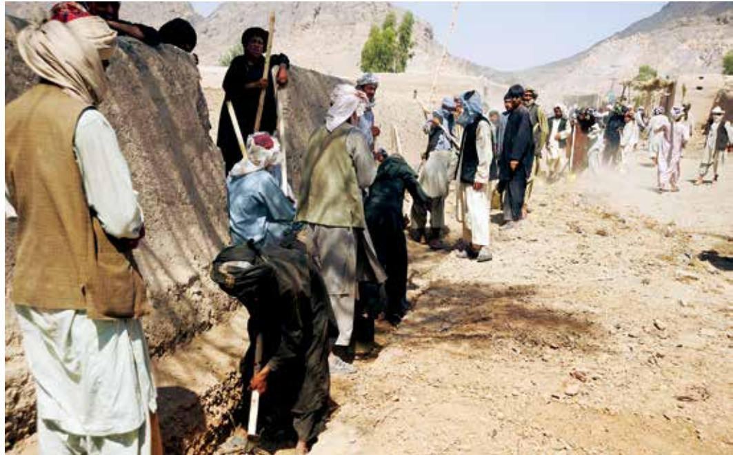
Afghans work on a road construction project in Spin Zurat village, Dand District, Kandahar Province, on June 22, 2010. (U.S. Air Force photo by Technical Sgt. Joselito Aribuabo)
