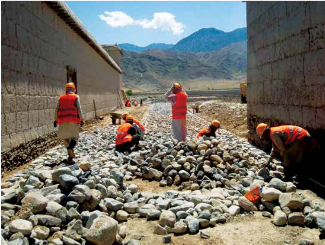
CCI-funded road construction in Sarkani District, Kunar Province, during summer 2013. (USAID photo)
