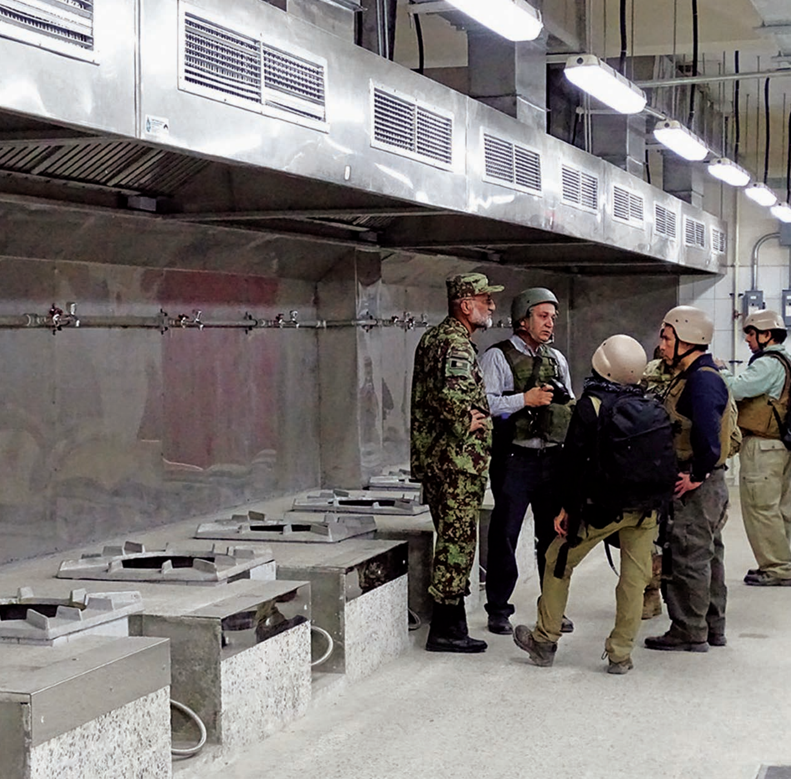
SIGAR inspects kitchen facilities at the Kabul Military Training Center. (SIGAR photo)
