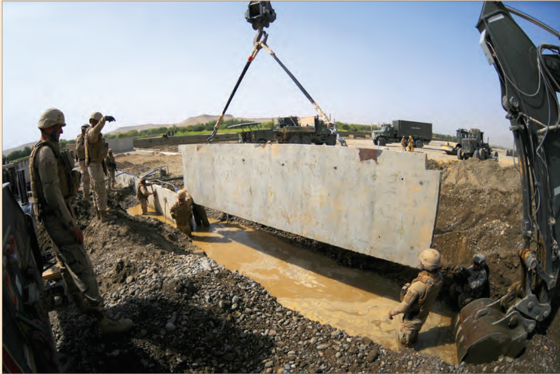
U.S. Seabees place prefabricated concrete pieces in the riverbed at the Musa Qal'eh low-water-crossing project. (Navy Photo by Mass Communication Specialist 1st Class Russ Stewart)
