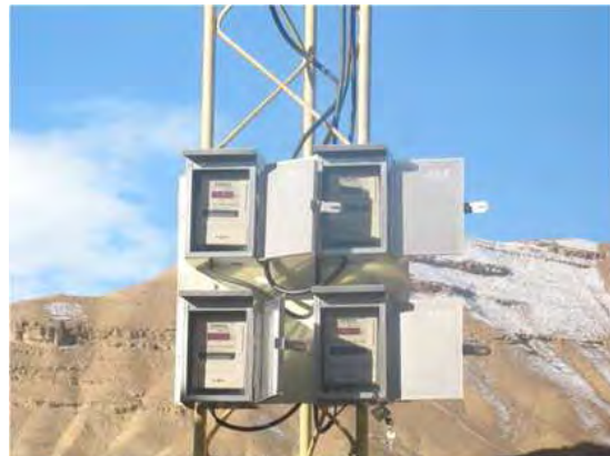
Photo 12 - Prepaid Meters for Household Consumption Monitoring
