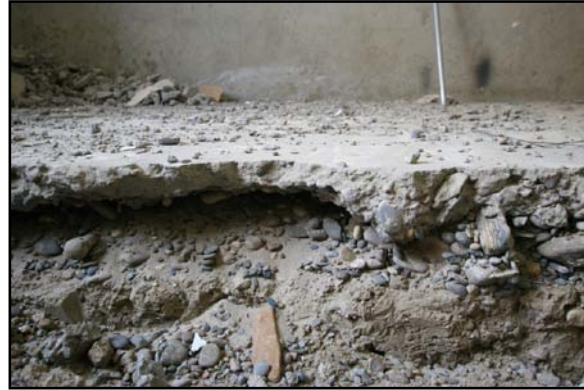
Photo 3: Poor Concrete Slab-on-Grade with No Reinforcement at Garm Ser Site
