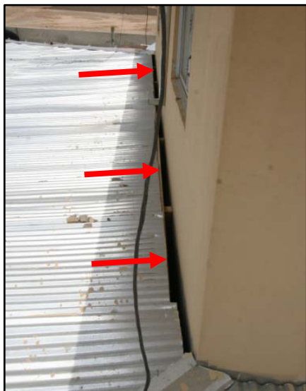
Photo 7: Gap Between Roof Panels and Exterior Wall at Nahri Saraj Site
