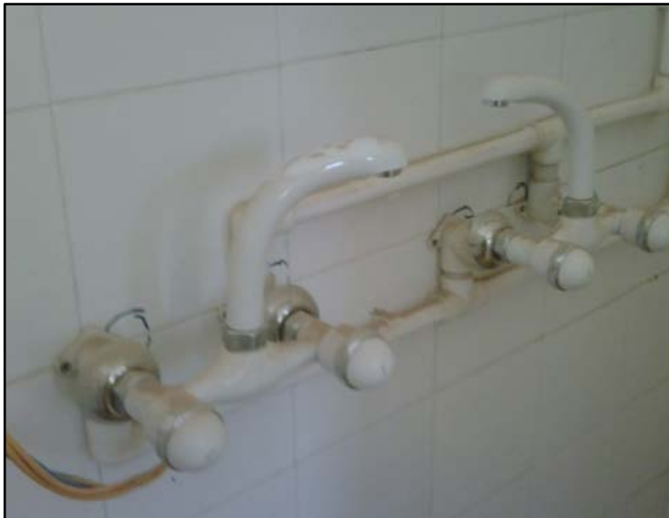
Photo 13: Residential Grade "Goose-Neck" Faucets at Takha Pul Site
