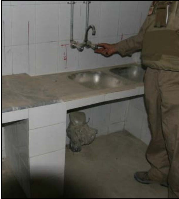
Photo 14: Residential Grade Undersized Scullery Sink at Nad Ali Site
