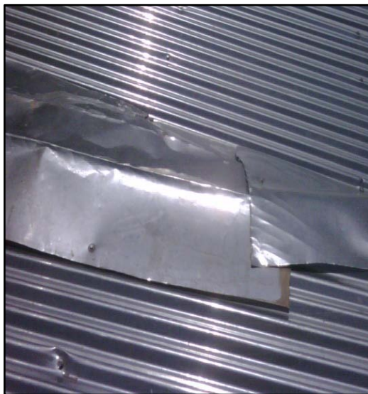
Photo 8: Damaged Roof Panels and Improper Flashing Installation at Spin Boldak Site
