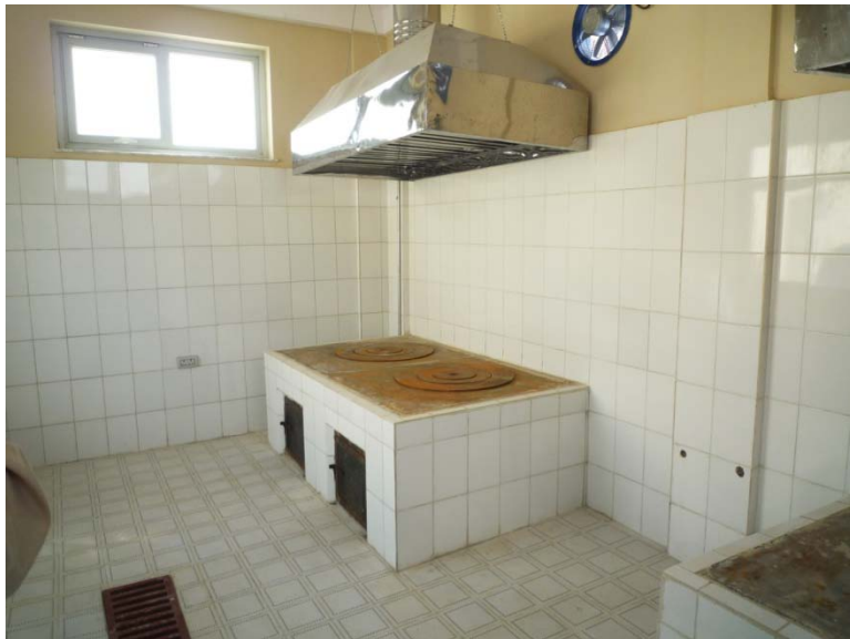
Photo 2: RLC Kitchen Stove and Exhaust Fan
