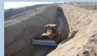
Photo: Anti-Vehicle and Flood Control Trench, Feb. 2010
