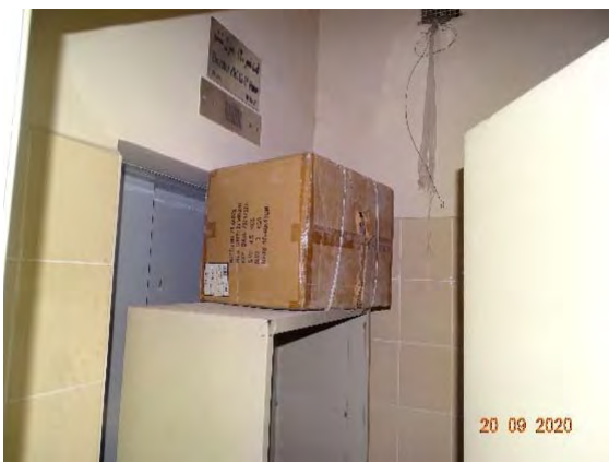
Photo 1 - Equipment Blocking Unused Elevator
