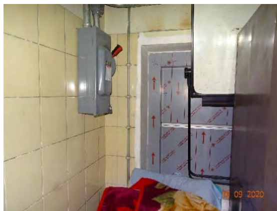
Photo 2 - Equipment Blocking Unused Dumbwaiter
