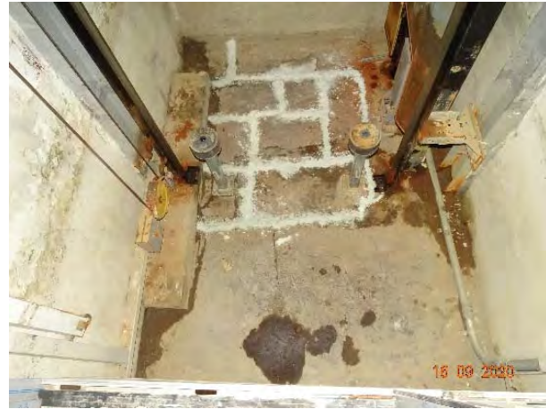
Photo 3 - Water Damage in Elevator Shaft
