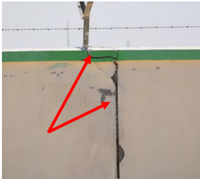
Photo 8 - Cracks in Boundary Wall
