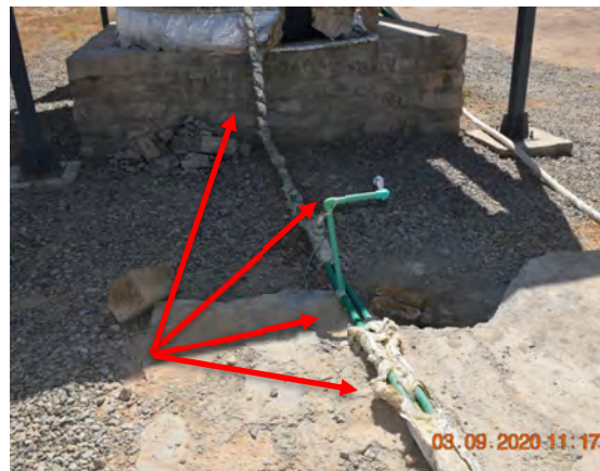
Photo 3 - Site Visit Photo With Prohibited Piping
