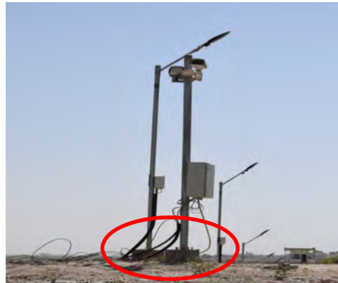
Photo 5 - Exposed Wiring Surrounding Pole Bases
