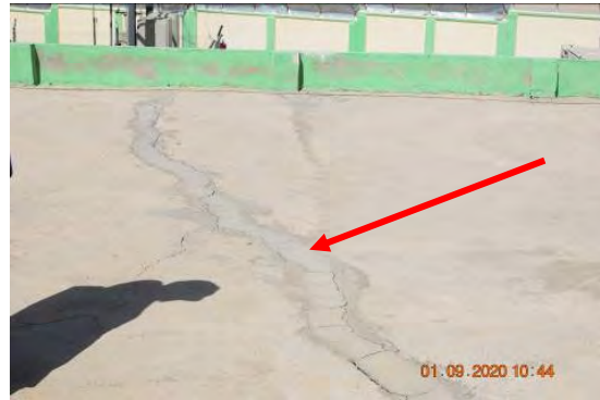
Photo 9 - Cracks in the Control Building's Roof
