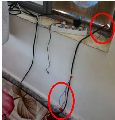
Photo 6 - Interior Exposed Spliced Wiring in Guard Tower
