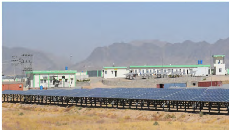
Photo 1 - Kandahar Solar Power Plant
