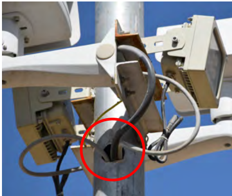
Photo 4 - Unsealed Opening in Pole
