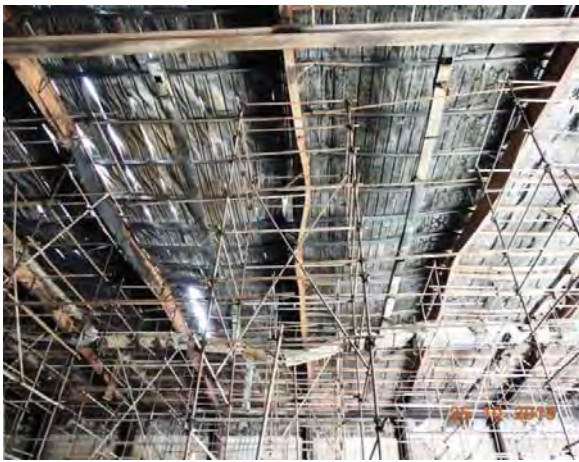
Photo 1 - Damaged Rafters in the JAF I Hangar
