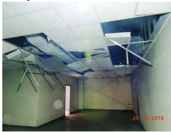
Photo 2 - Damaged Office Ceiling in the Attached Building
