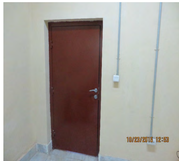
Photo 1 - Non-Fire-Rated Door Installed in Renovated Training Classroom Building 402
