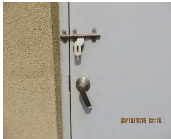
Photo 6 - East Side Exit Door Slide Locked from Outside
