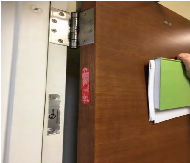
Photo 4 - Certified Fire Door Label Placed on Door and Doorframe
