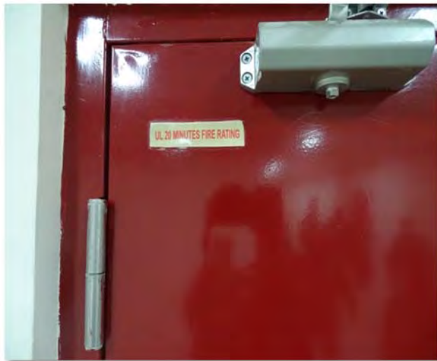
Photo 5 - Door at KMTC with Counterfeit UL Labels
