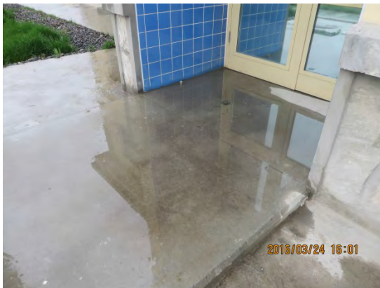
Photo 1 - Pooling Water in the MOI Headquarters Building Entrance
