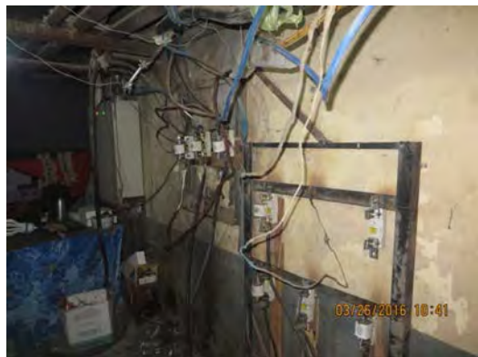
Photo 3 - Poorly Maintained Electrical Panel Board in Block 2 Office Building
