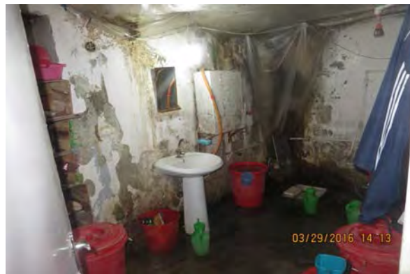
Photo 4 - Poorly Maintained Bathroom in Block 3
