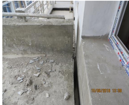
Photo 3 - Chipped Concrete Between Dormitory Building and Cafeteria Facility
