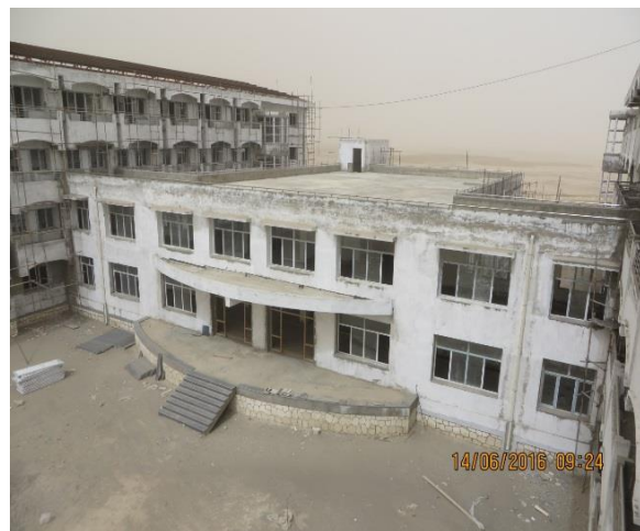
Photo 2 - Cafeteria Improperly Connected to Dormitory Buildings
