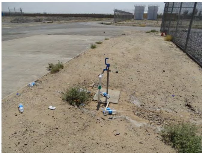
Photo 1 - Improperly Constructed Vehicle Wash Rack
