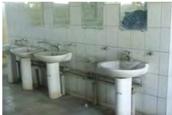
Photo 2 - Poorly Maintained Facilities in Bathroom Building 7
