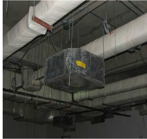
Photo 3 - Ceiling-Mounted Equipment and Mechanical Duct Work With No Lateral Bracing
