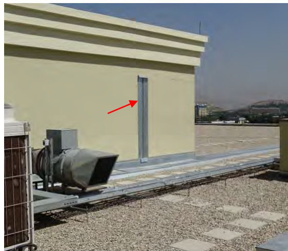
Photo 2 - Separation Joint Is Not Continuous at Top
